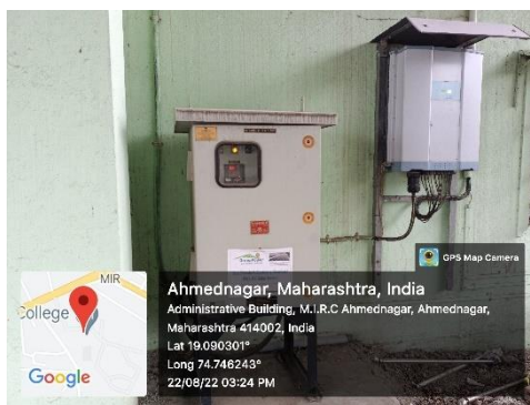
Figure 3: Drinking water filter system at every floor with cooler
